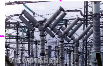
the electricity is stepped-down at a local power sub-station (8000 V)
